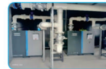
Vacuum energy-saving transformation
