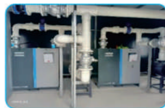
Vacuum energy-saving transformation
